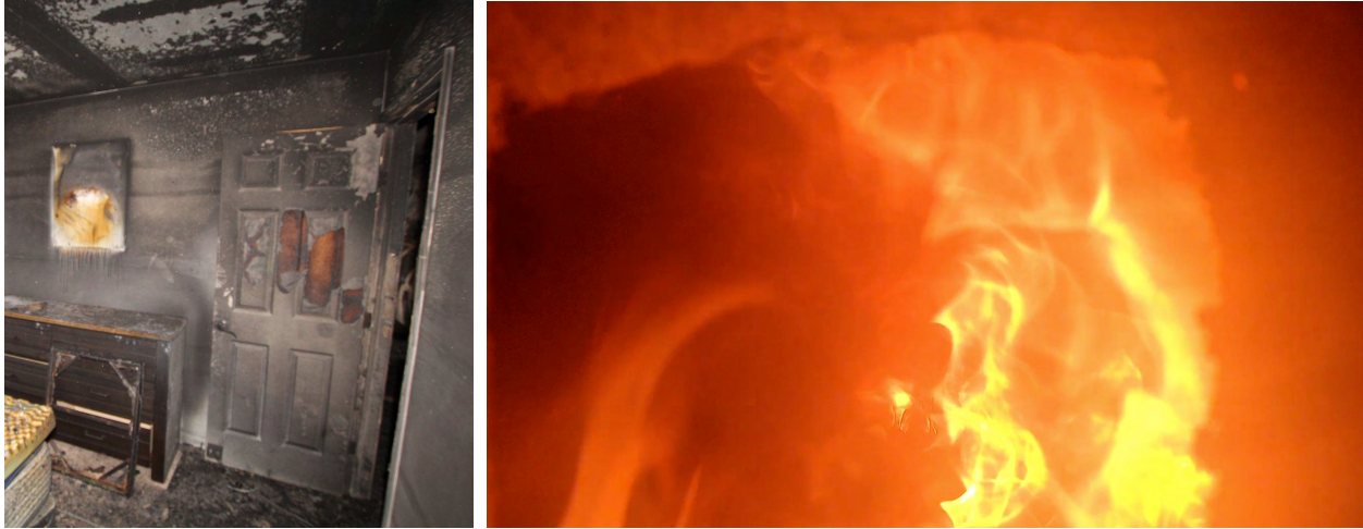
(a) Post-Suppression Bedroom 2 Door (b) End Hallway (Outside of Bedroom 2) Flame Spread Prior to Suppression
