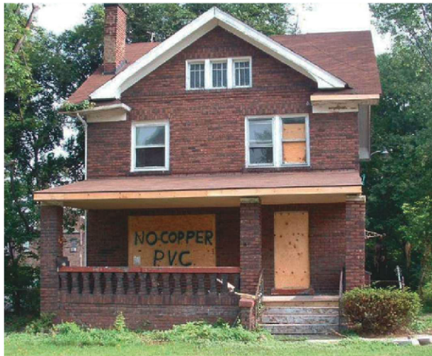
Many vacant buildings have been vandalized and “stripped out” of copper and other valuable metals. In such buildings, walls and floors may have been torn apart and fire will be able to spread quickly throughout the interior.
