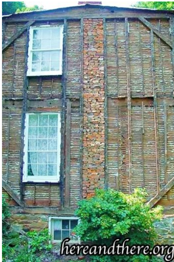
Example of balloon framing using full dimensional lumber. Note windows that are vertically aligned.
